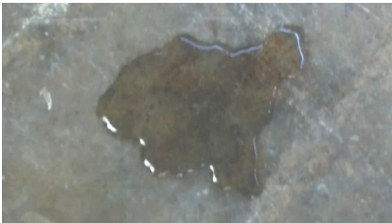
Non-absorbent Sub Floor
