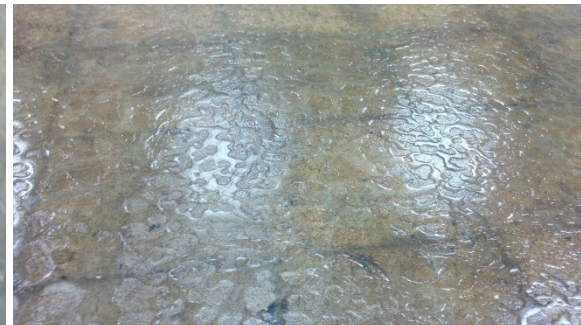
Result of contaminated Sub Floor
